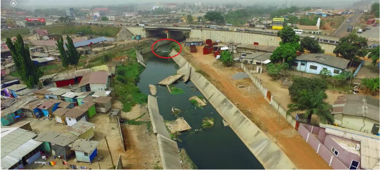
Fig. 1: Damaged sections of the lined Odaw River Channel at Achimota
