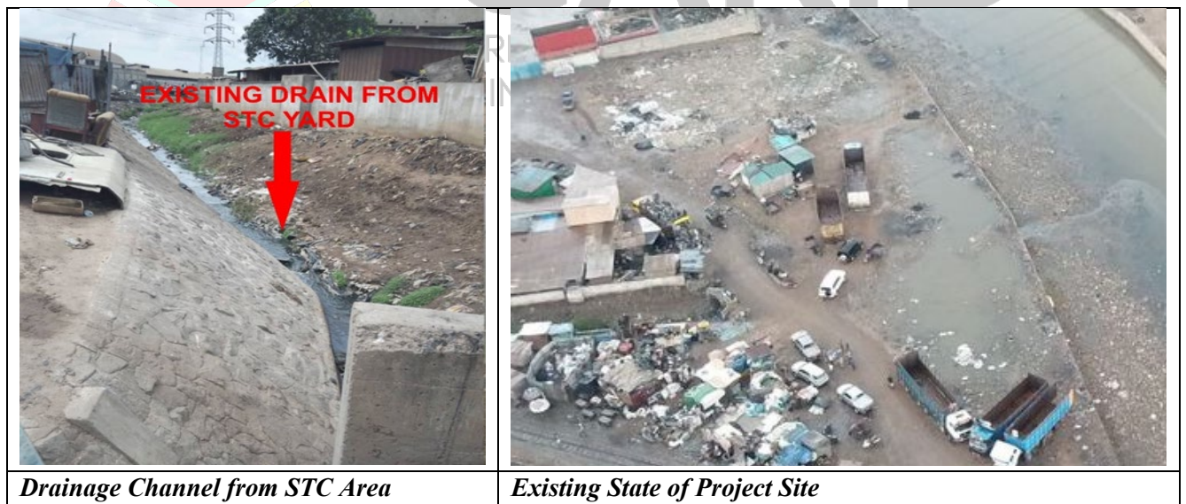
Figure 5.9 Drainage Condition at Odawna Site
