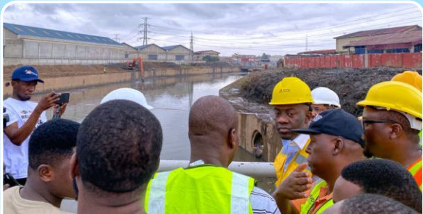
Hon. Kojo Nkrumah (in yellow reflective vest and yellow safety helmet) on inspection tour of the dredging site.
